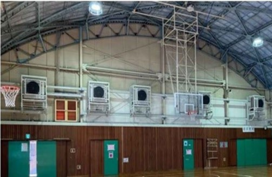
Example of air conditioning installation (indoor units)
