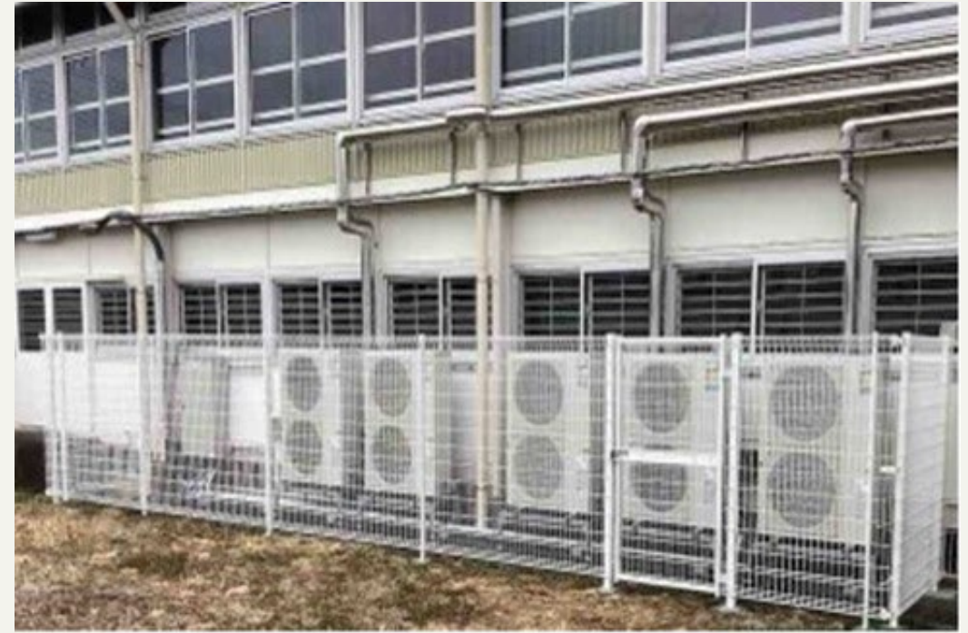
Example of air conditioning installation (outdoor units)
